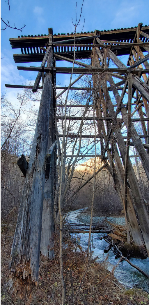
The wooden Gilahina trestle was originally 890 feet long and 90 feet high. It required one-half million board feet of timber and was completed in eight days in the winter of 1911. Due to the rugged landscape, over 15% of the entire railway was built on trestles like this. Photo by Dave Hollis.
